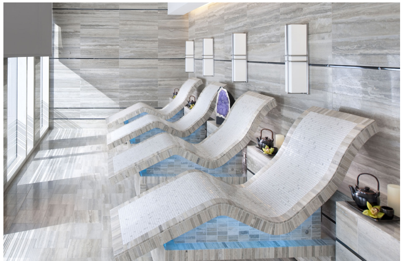
WarmlyYours TempZone™ installed in Mandarin Oriental Pool & Spa
